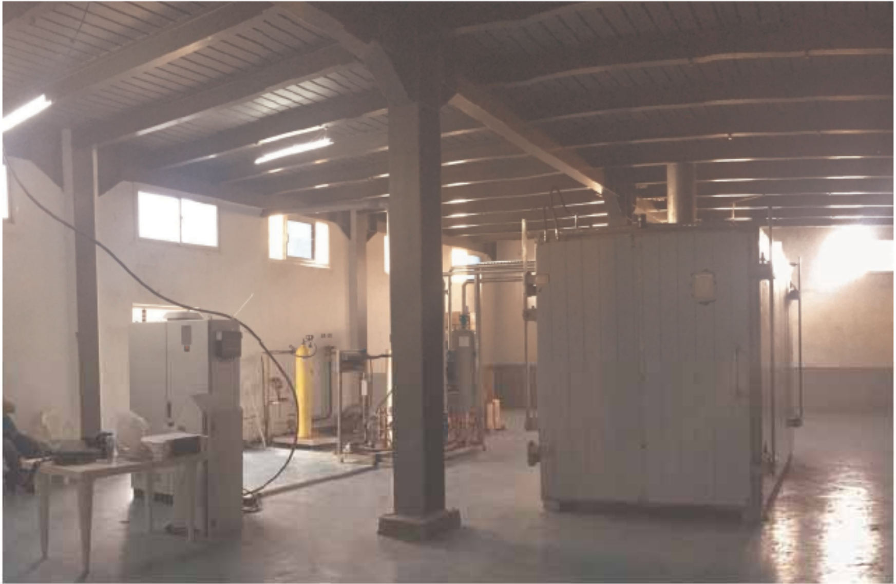
15 M3 ETO STERILIZER VIEW – DOUBLE DOOR – ELECTRICAL PANEL – KIOSK – MACHINE PARK
