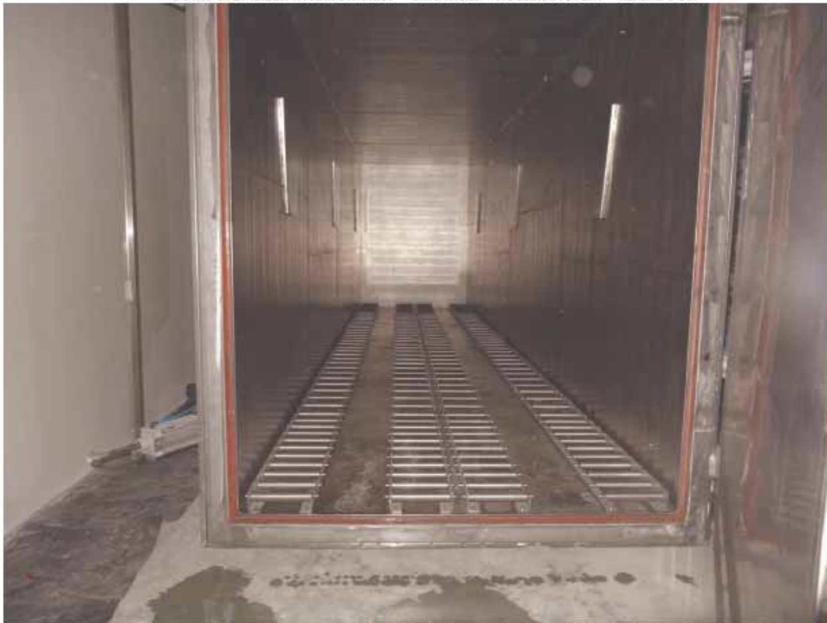
34 M3 STERILIZER INTERIOR VIEW – CHANNELS – ROLLER SYSTEM – REAR DOOR
