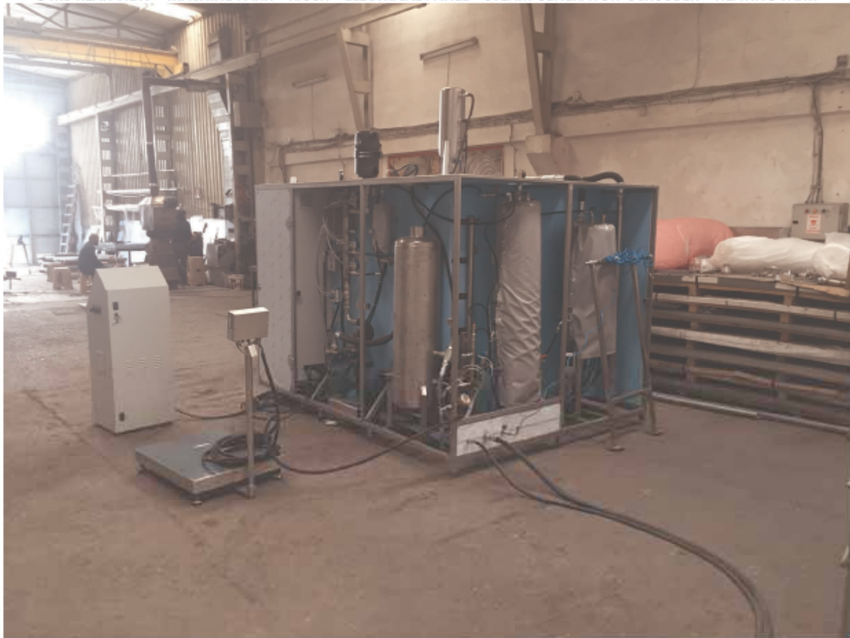
5 M3 REAR VIEW – MACHINE PARK – KIOSK – ELECTRICAL PANEL – STEAM GENERATOR- SCRUBBER – HEATING TANK
